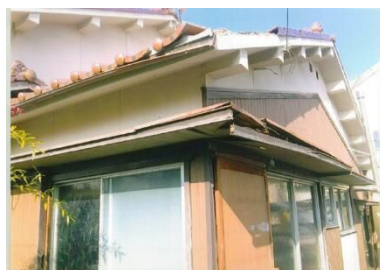
庇の腐朽・破損
